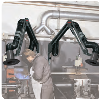
Extraction arm at a welding station
