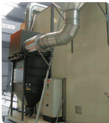
DUSTMAC filter unit on sanding station
