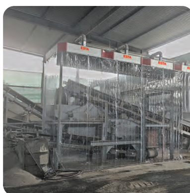
Extraction hoods over conveyor belts
