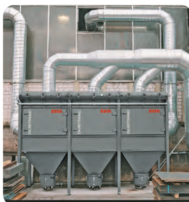
Modular filtration unit
