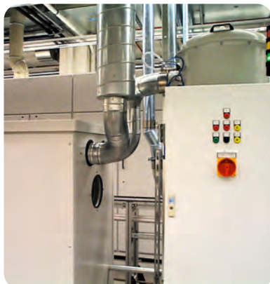
Control unit with monitoring lamps
